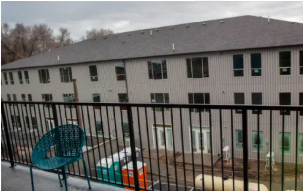
An affordable housing building under construction in January 2020 in Salt Lake City that is supported by the Utah Housing Preservation Fund. The three-story building will feature 21 units with three and four bedrooms. Source: Deseret News
