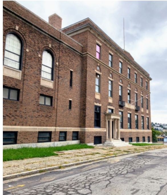
Creative Hub Worcester (CHW), the rehabilitation of a historic building in downtown Worcester and conversion to a community center serving an under-resourced community, with a focus on creative and cultural expression.
